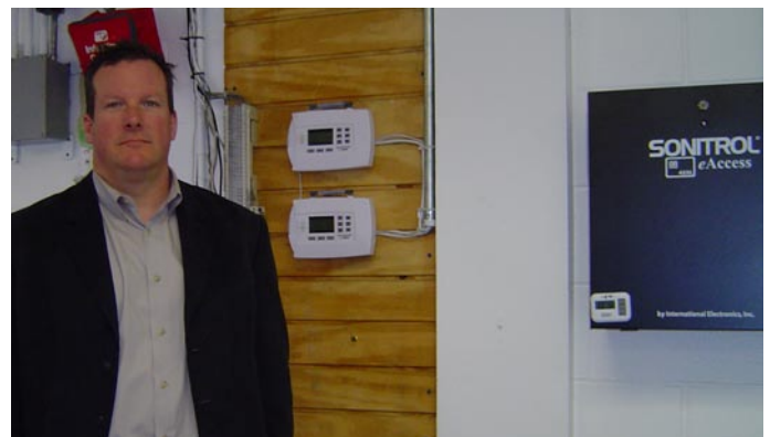
The EA800 output relays connect to the Sonitrol eAccess system.
